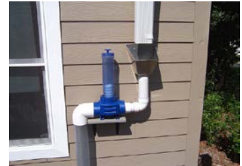
Rainwater collection system
