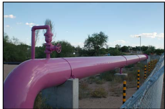
Reclaimed water distribution line
