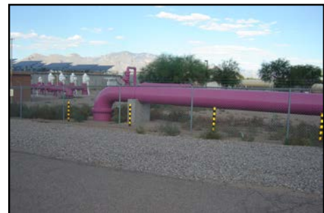
Purple irrigation pipes for treated effluent
