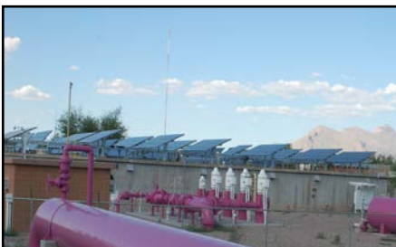
Photovoltaic solar panels
