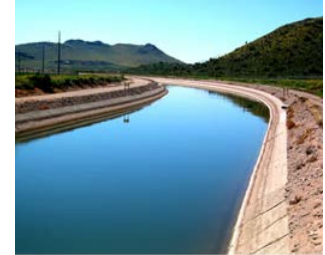
CAP distribution line
